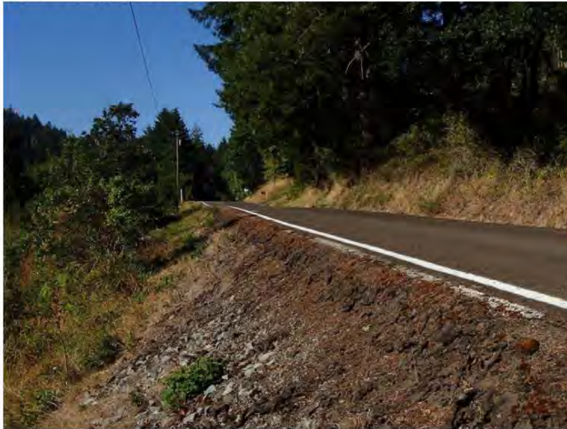
Figure 1 Drop-off at Edge of NW Oak Creek Drive
