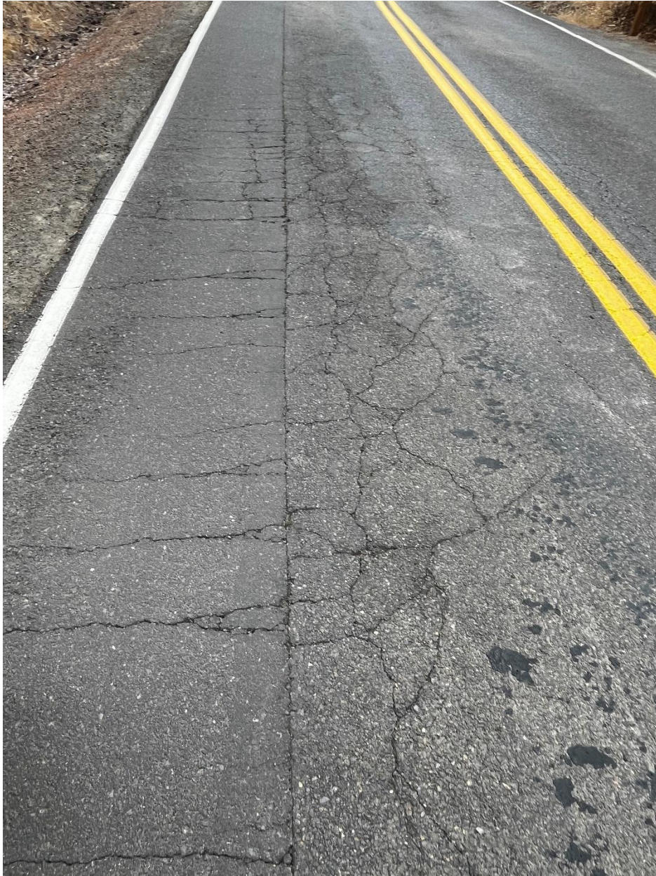
Additional documentation of degradation of Powers Ave.
