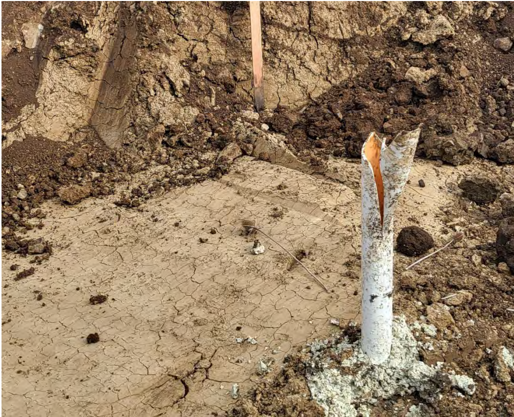
Photo A-1 – Well casing of damaged original piezometer P-9.
