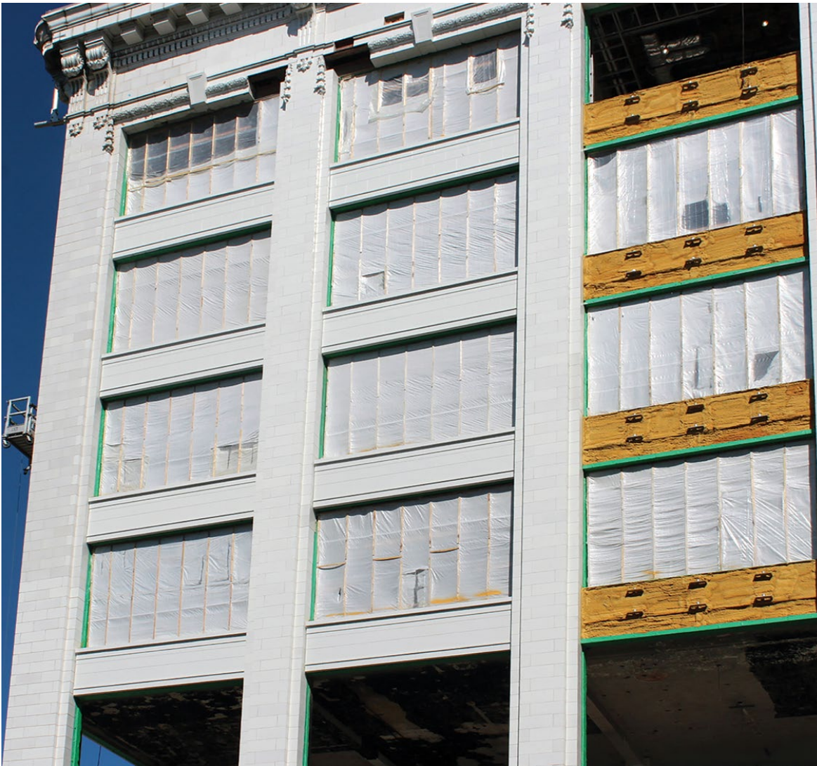
Figure 18. Missing historic terra cotta spandrel panels on all floor levels were recreated utilizing glass fiber reinforced concrete (GFRC) replacements. New spandrels were fabricated as individual components and attached with metal clips between historic terra cotta piers. Photo: Kris Frail, Dewberry.
