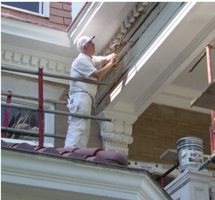
[12] Repair and limited replacement in kind to match deteriorated wood porch features is always a recommended preservation treatment.
