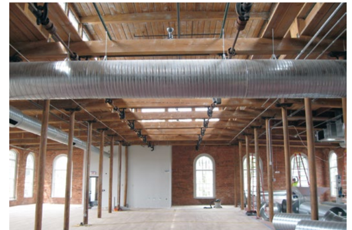
[39] Leaving the ceiling structure exposed and installing exposed ductwork where it does not impact the windows, are appropriate treatments when rehabilitating an industrial building for another use.
