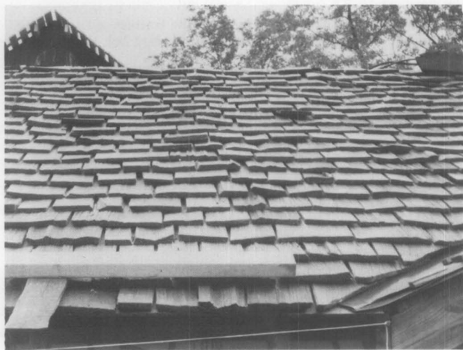
15. These commercially available roofing products with rustic split faces are not appropriate for historic preservation projects. In addition to the inaccurate appearance, the irregular surfaces and often wide spaces between shingles will allow wind-driven moisture to penetrate up and under them. The excessively wide boards will tend to cup, curl and crack. Moss, lichens and debris will have a tendency to collect on these irregular surfaces, further deteriorating the roofing. Photo: Sharon C. Park.
