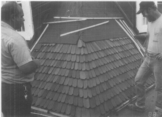
D. The fanned hips (seen here), swept valleys, and projecting ridge combs were installed as part of the re-roofing project. Special features, when documented, should be reproduced when re-shingling historic roofs.
