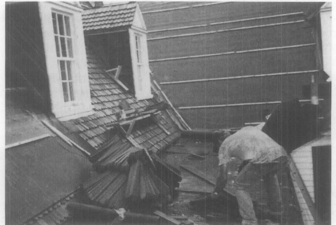
C. The replacement shingles (see specifications above), matched the historic shingles and were of such high quality that little hand dressing was needed at the site. The building paper, a temporary protection, was removed as the shingles were installed on the sheathing boards.
