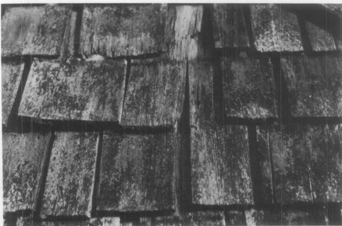
16. Routine maintenance is necessary to extend the life of the roof. On this roof, the shingles have not seriously eroded, but the presence of lichens and moss is becoming evident and there are a few cracked and missing shingles. The moss spores should be removed, missing shingles replaced, and small pieces of metal flashing slipped under cracked shingles to keep moisture from penetrating. Photo: Williamsport Preservation Training Center.
