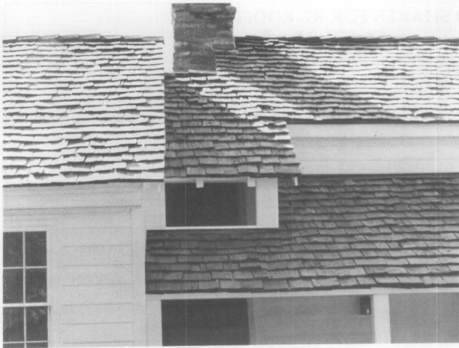
12. Inappropriately selected and installed wooden shingles can drastically alter the historic character of a building. This tavern historically was roofed with handsplit and dressed shingles of a relatively smooth appearance. In this case, a commercially available shake was used to effect a "rustic" appearance. Photo: National Park Service.
