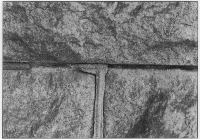
Figure 8. Due to inadequate joint preparation, the repointing mortar has not adhered properly and is falling out of the joint. Photo: Robert C. Mack, FAIA.
