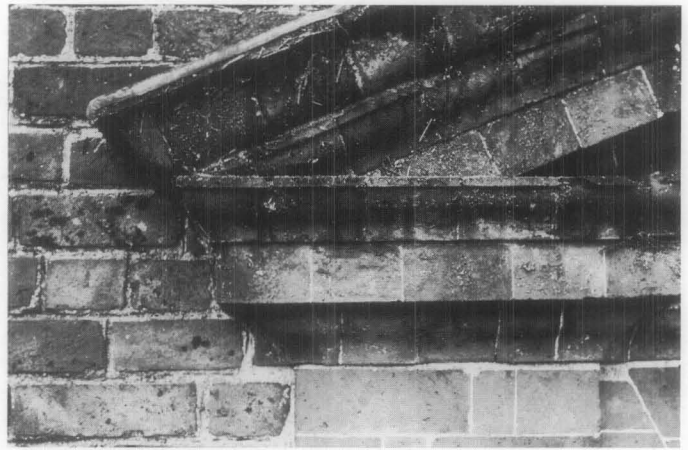
Figure 19. Mortar joints of 18th century brick buildings were often as much as 1/2 inch wide, cut flush and struck with a grapevine joint, but for window and door surrounds where a finer quality rubbed brick was used, mortar joints were very thin. Photo: National Park Service Files.
