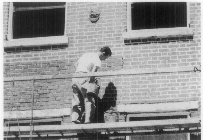
Figure 17. This photograph shows the significant visual change to the character of this historic brick building that has resulted from improper repointing procedures and a noticeably increased thickness of the mortar joints. Photo: Lee H. Nelson, FAIA.
