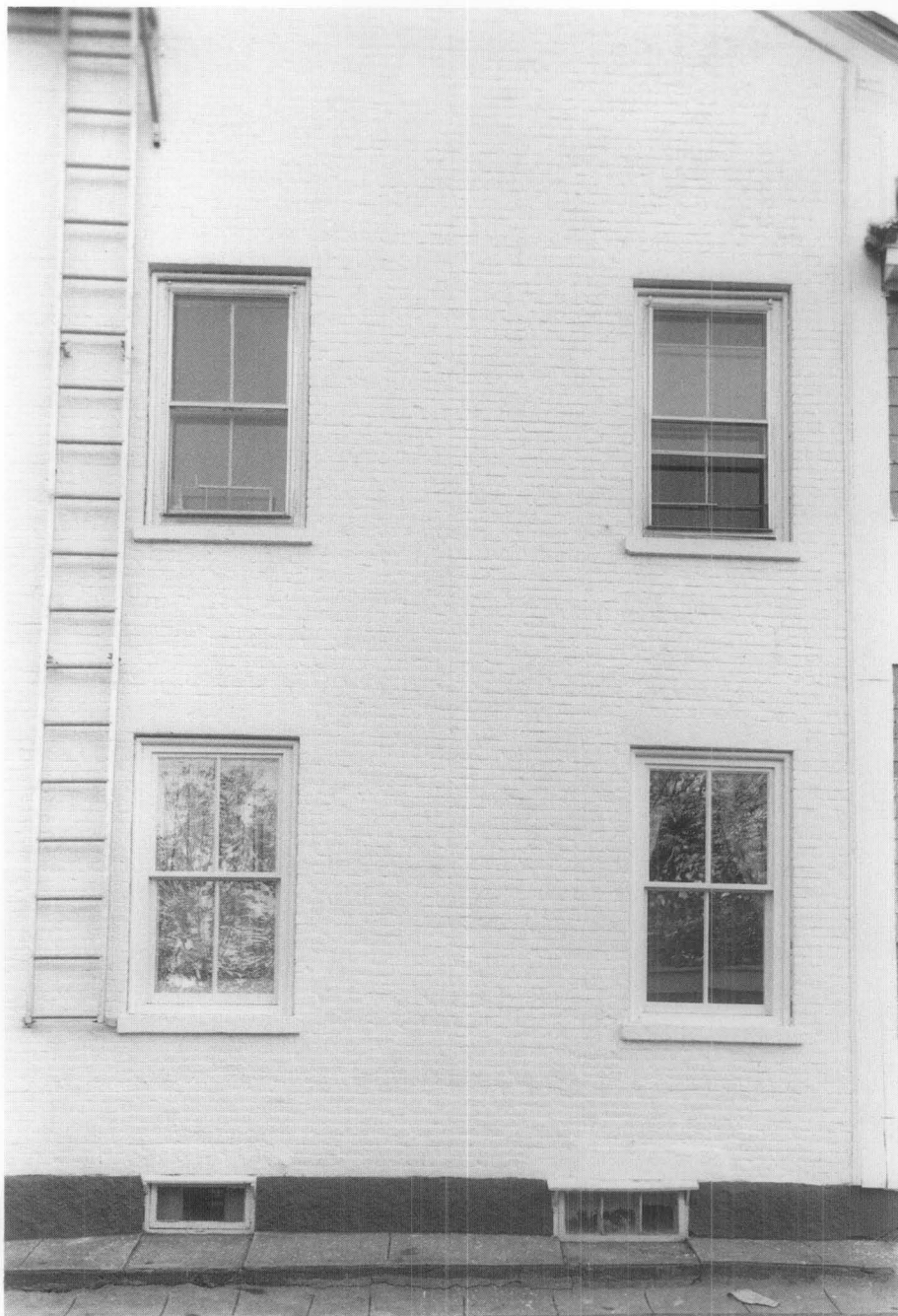
Figure 4. The new wooden windows on the first floor with insulating glass installed closely matched the historic windows which were preserved on the upper floor. Photo: Charles Parrott
