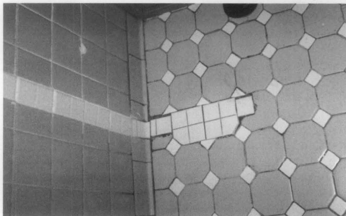
Figure 23. These non-matching tiles are inappropriate replacements for original tiles that were damaged during bathroom remodeling. Photo: Anne Grimmer.
