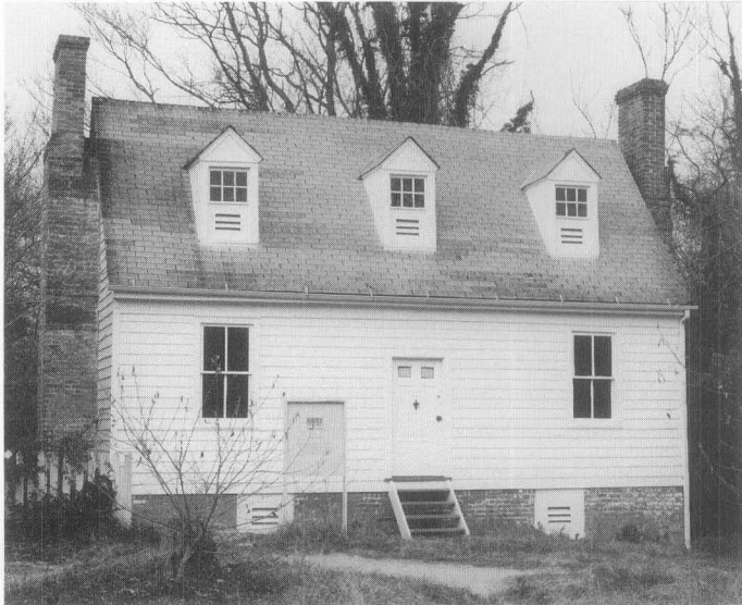
Figure 10. Regrading around the Booker Tenement at Colonial Williamsburg has protected the masonry foundation wall from excessive damp. This building has been successfully mothballed for over 10 years. Note the attic and basement vents, the temporary stairs, and the informative sign interpreting the history of this building.
