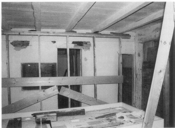
Figure 6. Interior bracing which will last the duration of the mothballing will protect weakened structural members. Jethro Coffin House. Photo: John Milner Architects.
