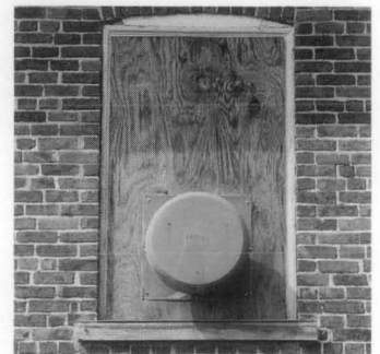
c. The exhaust fan has tamper-proof housing.
