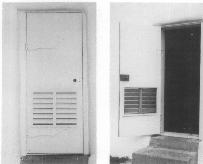
Figure 13. If historic doors would be damaged by adding extra locks, they should be removed and stored and new security doors added. At this lighthouse, the historic door has been replaced with a new door (seen both inside and outside) with an inset vent and new deadbolt locks. The heavy historic hinges have not been damaged. Photo: Williamsport Preservation Training Center, NPS.
