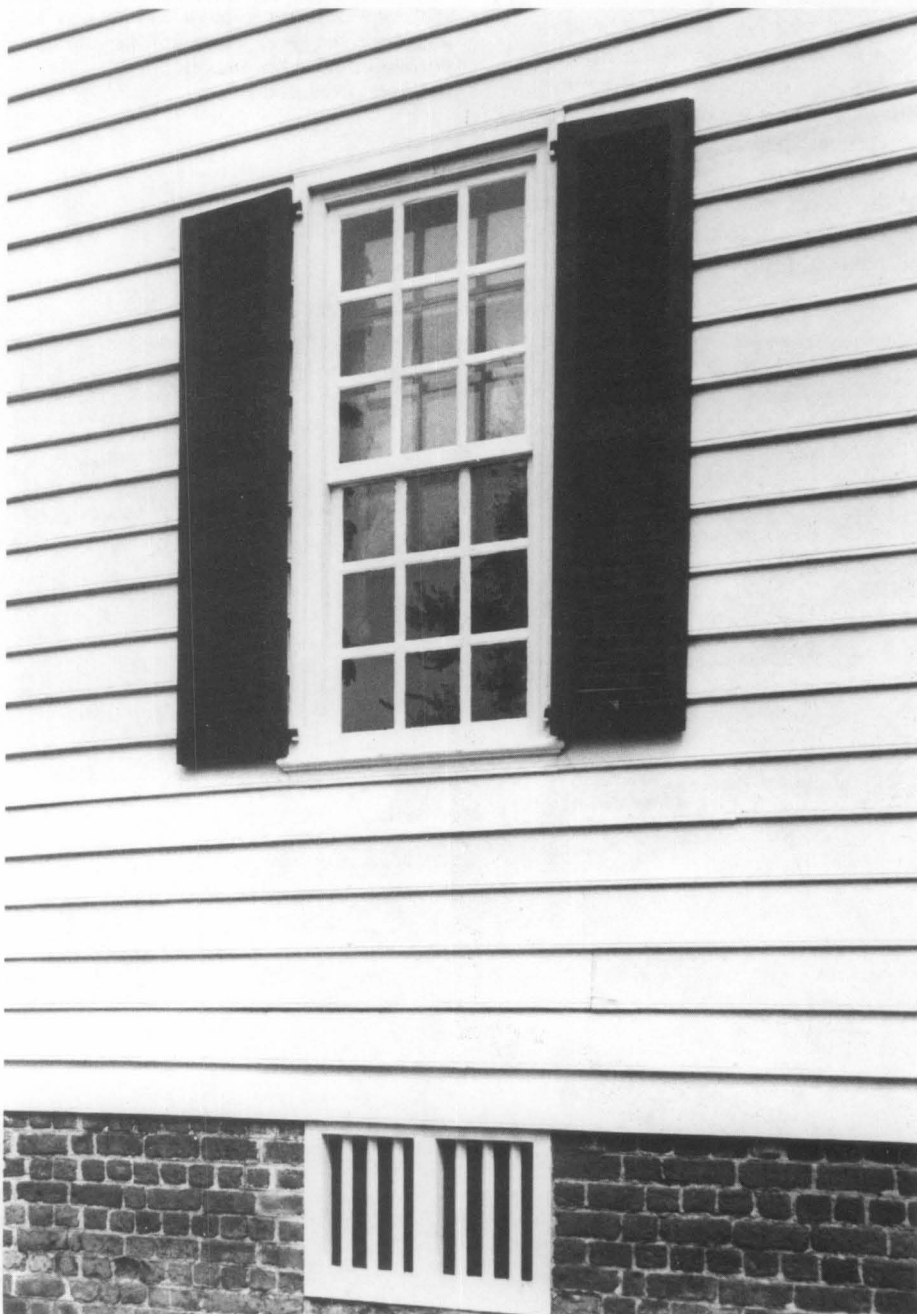
Figure 8. The unobtrusive interior storm window required no physical damage or exterior visual alteration to the original window. Photo: Tom H. Taylor.
