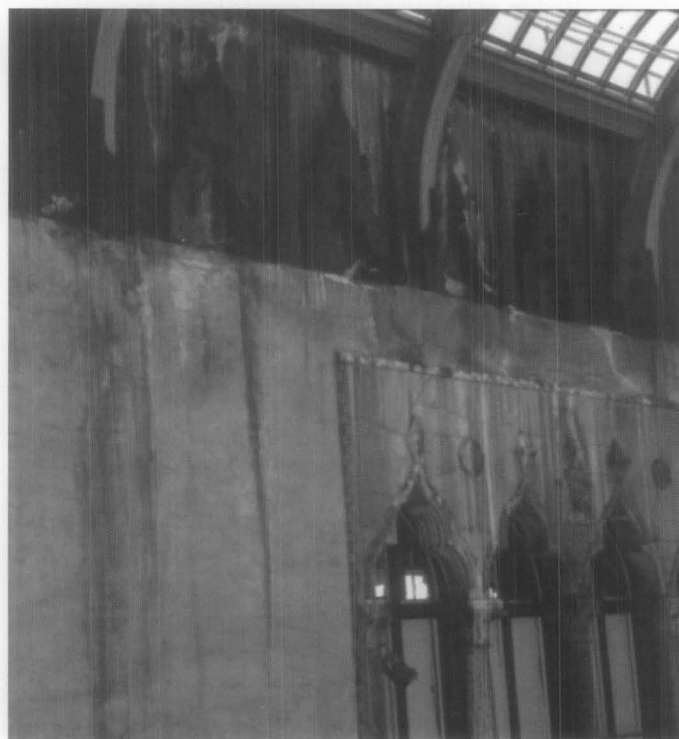
Fig. 7. Condensation dripping from the large overhead courtyard skylight was damaging the masonry in this museum. A new skylight with thermal glazing was installed, replacing the deteriorated single-glazed unit. A new climate control system monitors interior temperature and humidity. Photo: © Isabella Stewart Gardner Museum, Boston.
