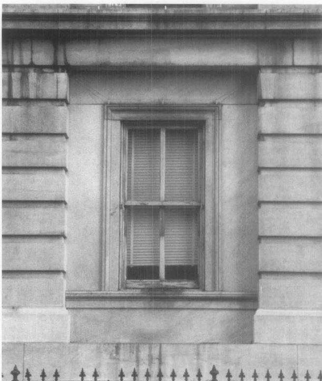
Fig. 10. Infiltration of damp air can occur around loose-fitting or deteriorated window sash and through cracks or open joints in building exteriors. Photo: Ann Brooks Prueher.
