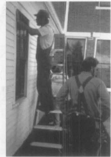
B. Repair exterior surfaces, paint, and recaulk as needed. Photo: Williamsport Preservation Training Center (WPTC), NPS.
