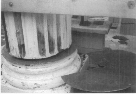
A. This lead sheet was installed at the base of the replacement column to stop rising damp. Photo: Bryan Blundell.
