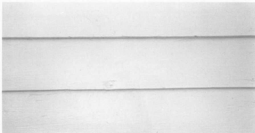
Figure 6. A typical section of the finish painted siding shows that little damage was done in removing the paint. Photo: Michael Lee
