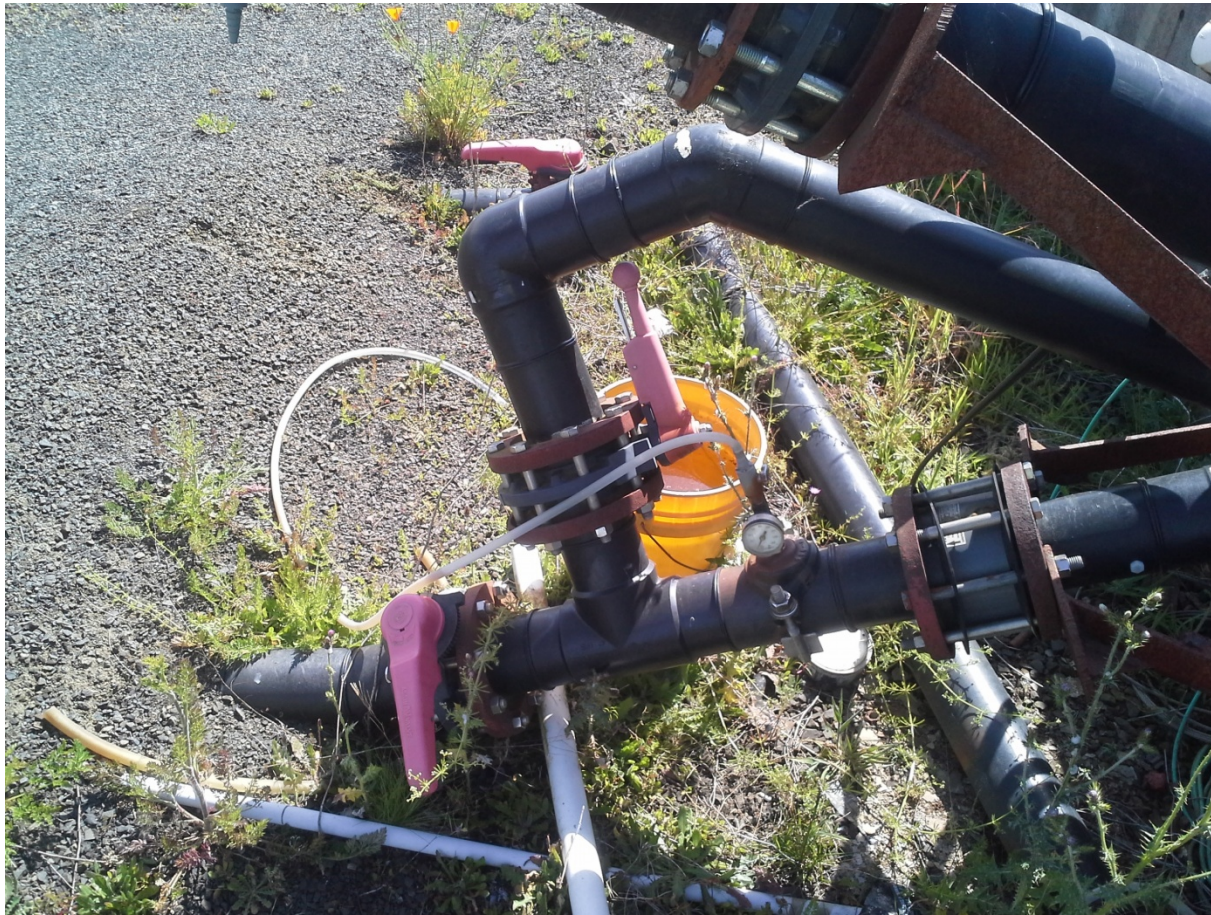
Sampling Port and Tubing at West Leachate Pond (L-Pond)
