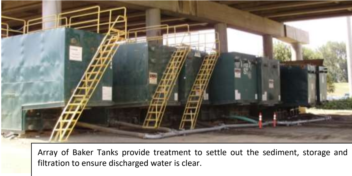
Figure 3-36 Array of Baker Tanks
