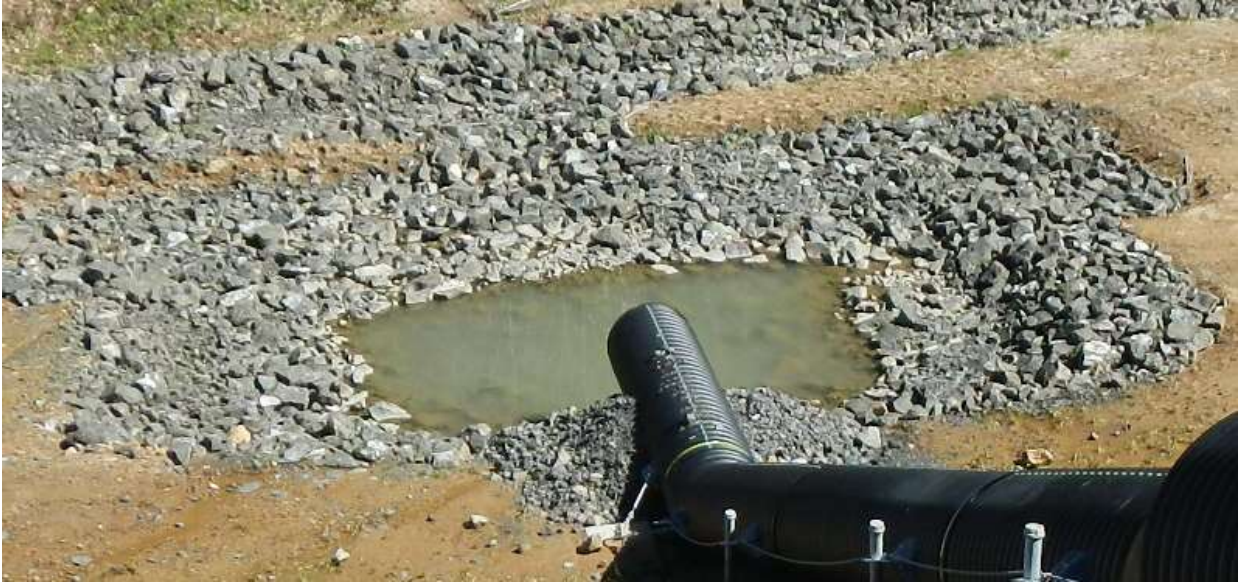
Figure 3-16 Energy Dissipater (permanent installation)
